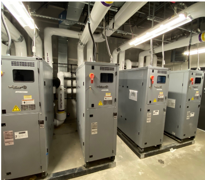
TruClimate 100 Water-To-Water Heat Pumps met every performance, energy, and decarbonization need identified by the school board.
